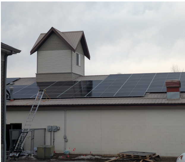
Photo: Solar installation in Ashby, Minnesota.
