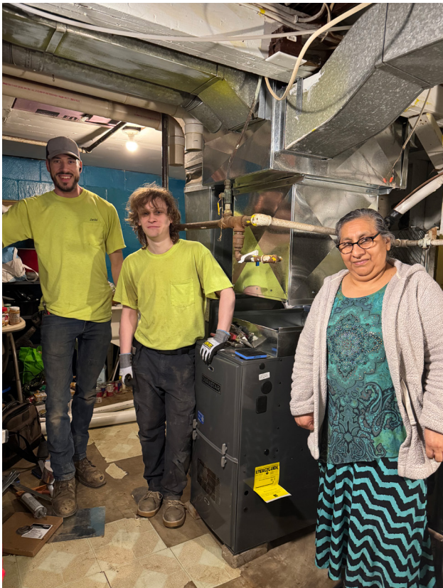
Photo: 96% efficient furnace installed in St. James.
