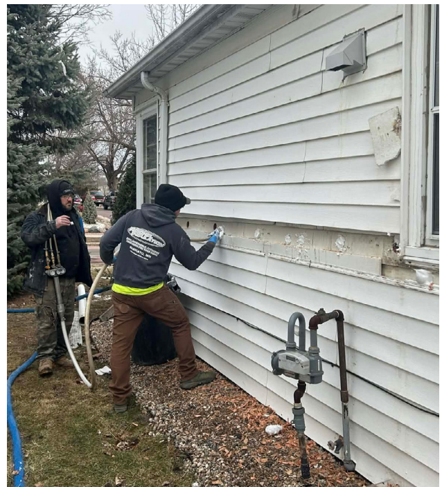
Photo: Insulation being installed to increase the energy efficiency of a home in St. James.
