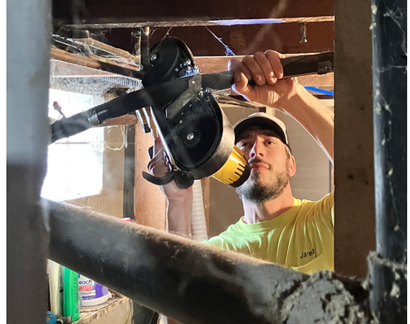
Photo: Jared Montagne of St. James Electric removing a gas line to install an all electric heat pump water heater.
