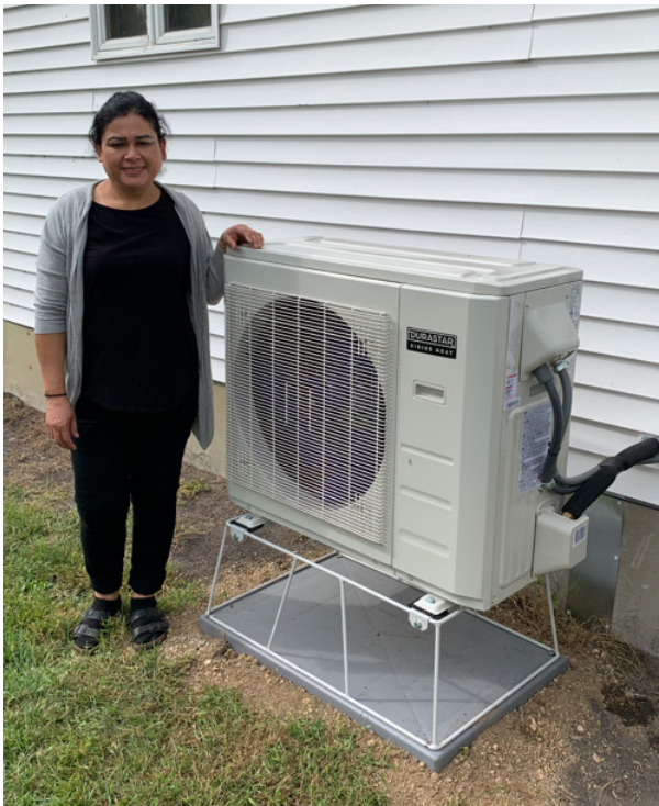
Photo: Air source heat pump installed in St. James.
