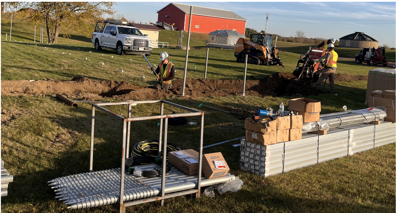
Photo: Solar installation in Comfrey, Minnesota.
